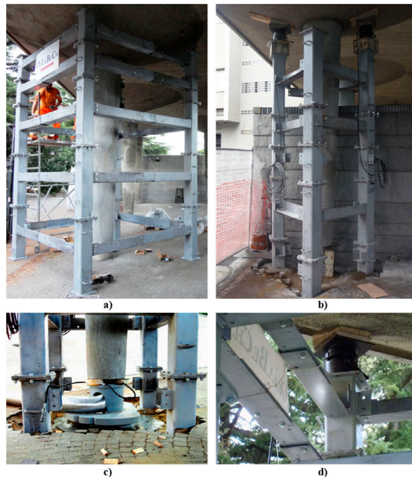
Figure 10. Different lifting steel frames: (a,b) the four- and three-columned ones, respectively, (c) base detail of the lifting frame, and (d) adjustment of the hydraulic jack head on the inclined surface of the mushroom column.
