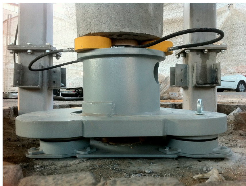
Figure 19. Picture of one of the tripods during its loading by means of three hydraulic jacks.
