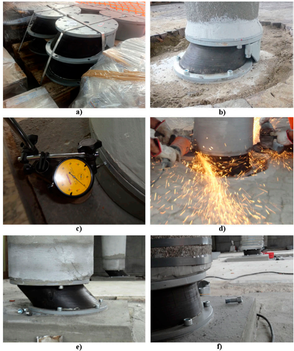
Figure 14. Some pictures of the pre-deformed LRB isolators: (a) storage of the devices at the construction yard; (b) pre-deformed LRB installed under the column; (c) installation of the high precision displacement transducer; (d) removal of the temporary constraint; LRB device at (e) the beginning, and at (f) the end of the re-centering operations.
