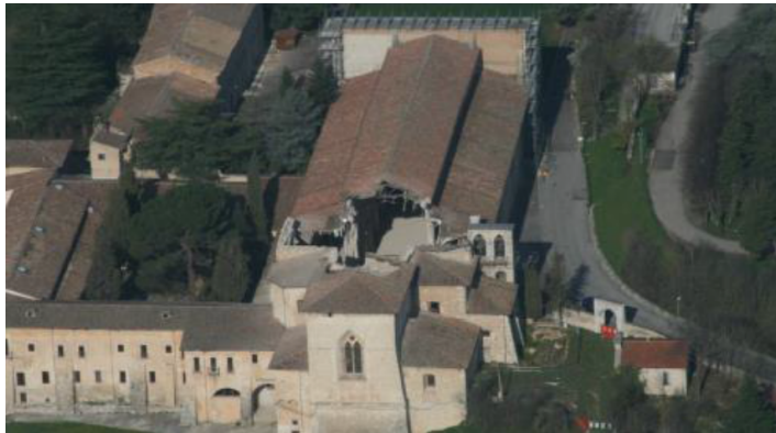
Figure 5.2. Collapse of the roof in the transept area following the 2009 earthquake.
