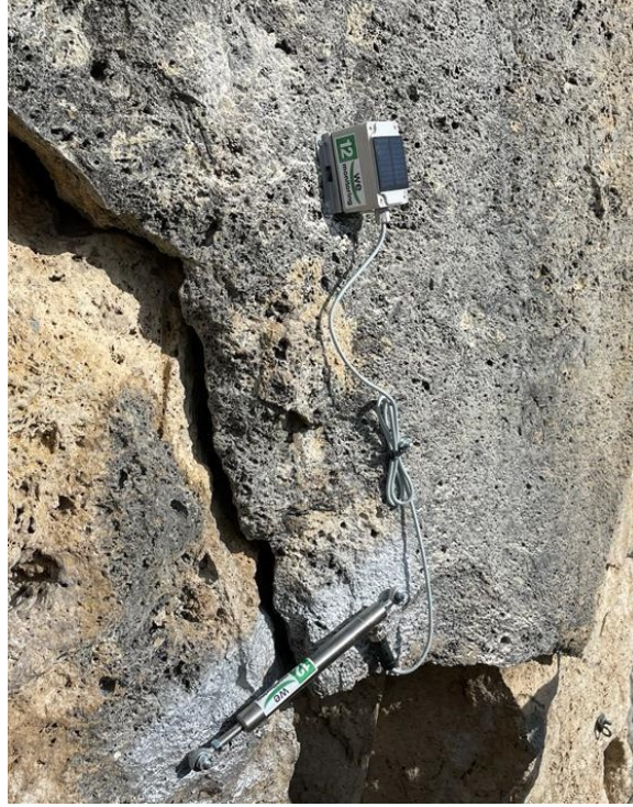
Figure 2.13. Implementation of the reported system with crack meters for rockfall monitoring [98].
