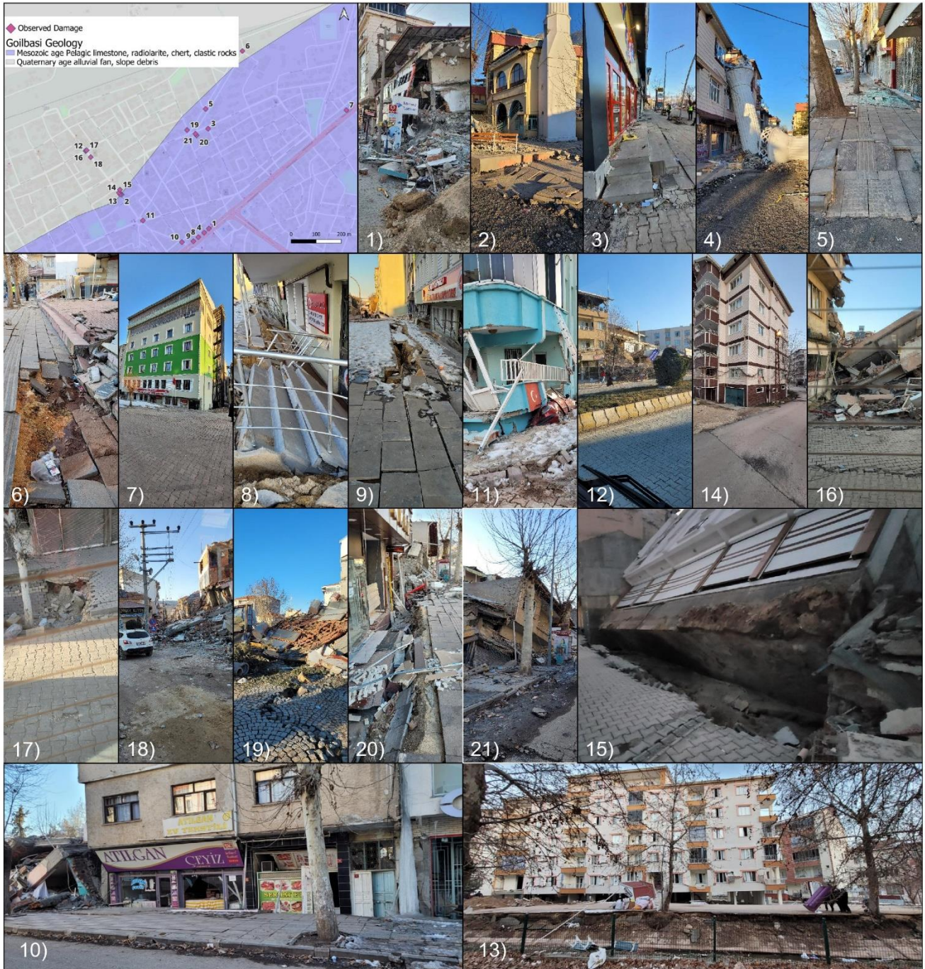
Fig. 10. Observed building damage due to liquefaction as collected in the field reconnaissance performed by the Turkish author in Gölbaşı.
