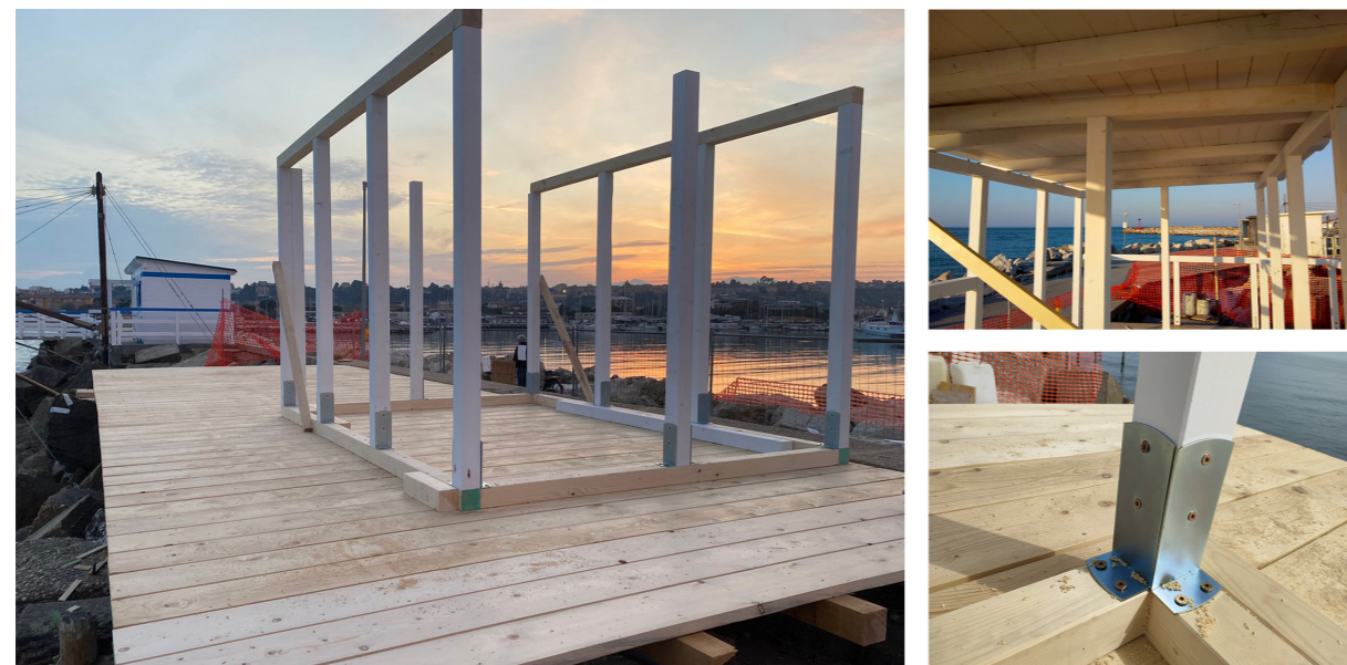
Fig. 7 - Construction of the shake and canopy structure, after laying the pier (Marchionni C. 2022).
