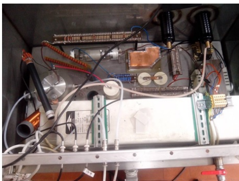
Figure 12. High Voltage system
