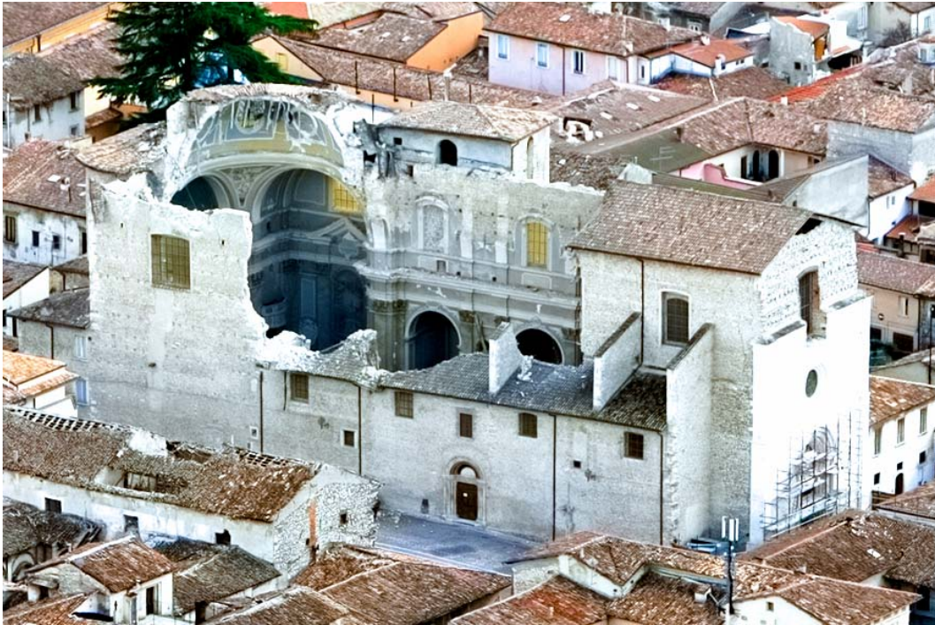
Figure 1. Church of Santa Maria Paganica after the 2009 earthquake (photo available online).
