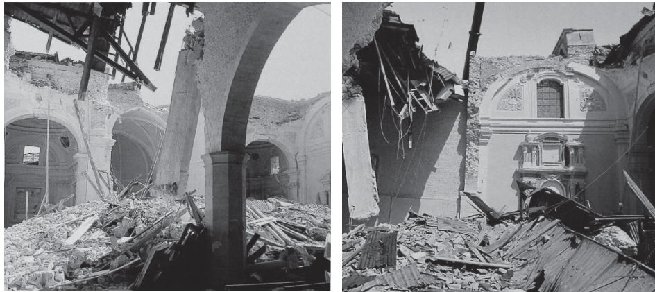
Fig. 5.13 – Fig. 5.14 The collapsed area of Collemaggio with the reinforced concrete elements hanging.
