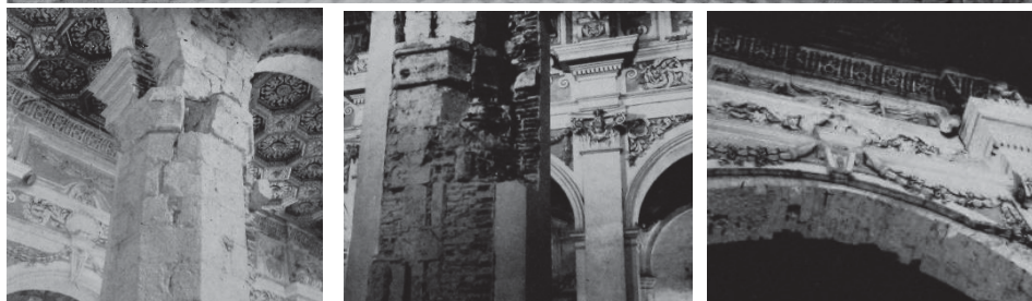
Fig. 3.55 – 3.56 – 3.57 Interior of Collemaggio before the intervention of Moretti. Details of the removal of the baroque stuccos.
