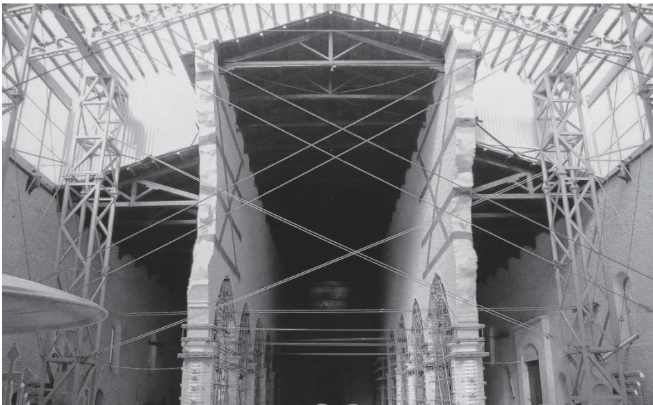
Fig. 5.20 Interior of Collemaggio with the provisional structures after the earthquake; view from the transept. It is possible to see the top beam in reinforced concrete on the left, at "middle height" of the wall of the main nave.
