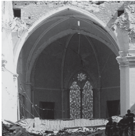
Fig. 5.15 – left The collapsed transept areas with the hollow elements in the masonry due to the falling of top beams.
