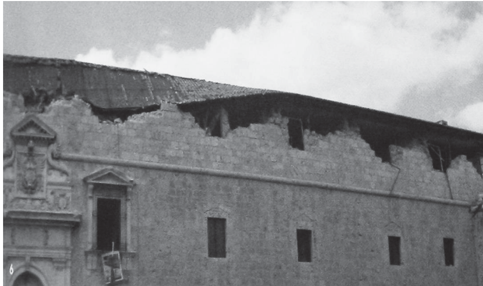
Fig. 5.2 Damages on the Castle of L'Aquila after 2009 quake event. The top beams pushed out of the plane the masonry.
