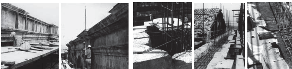
Fig. 3.31 - 3.32 - 3.33 Realization of the top beam and connection to the column of the facade: positioning of the connecting bars, positioning of the bond beam bars, pouring of the concrete.
