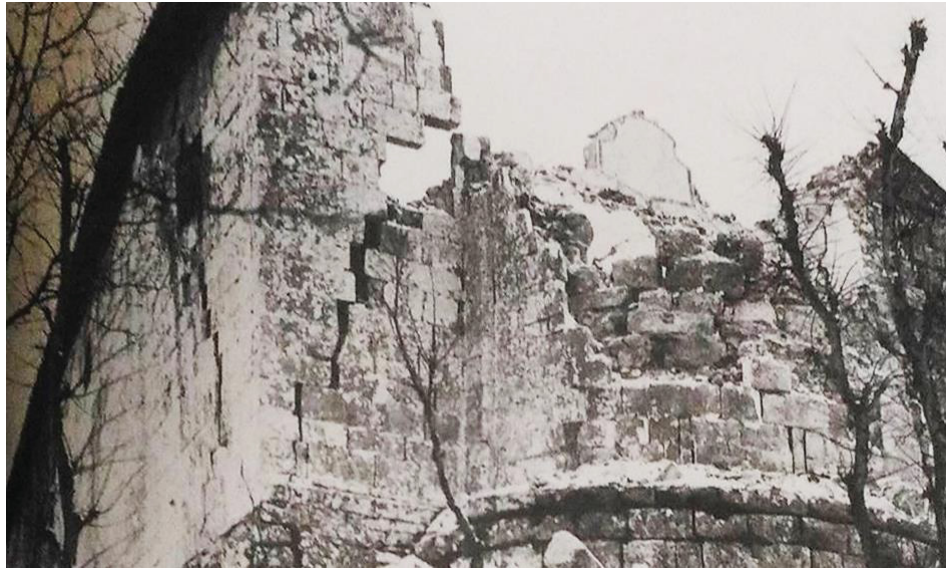
Fig. 3.64 View of the apse collapsed with the earthquake.
