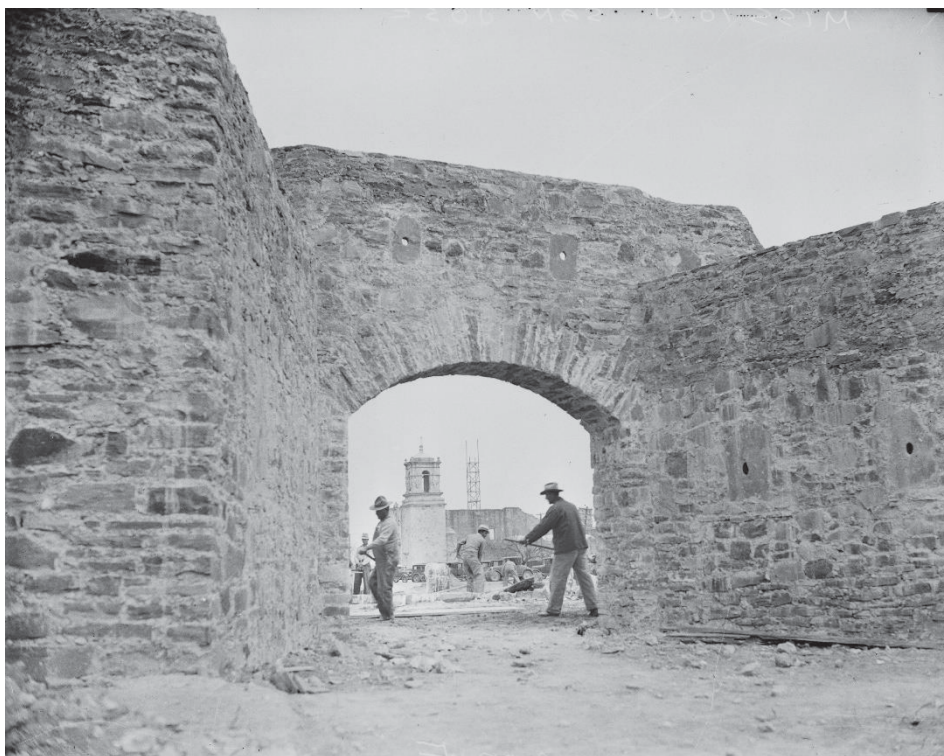
Fig. 4.51 Fortified gate constructed by Civil Works Administration employees from plans by restoration architect Harvey Smith, February 1934. It is possible to see the bell tower reconstructed. (UTSA)
