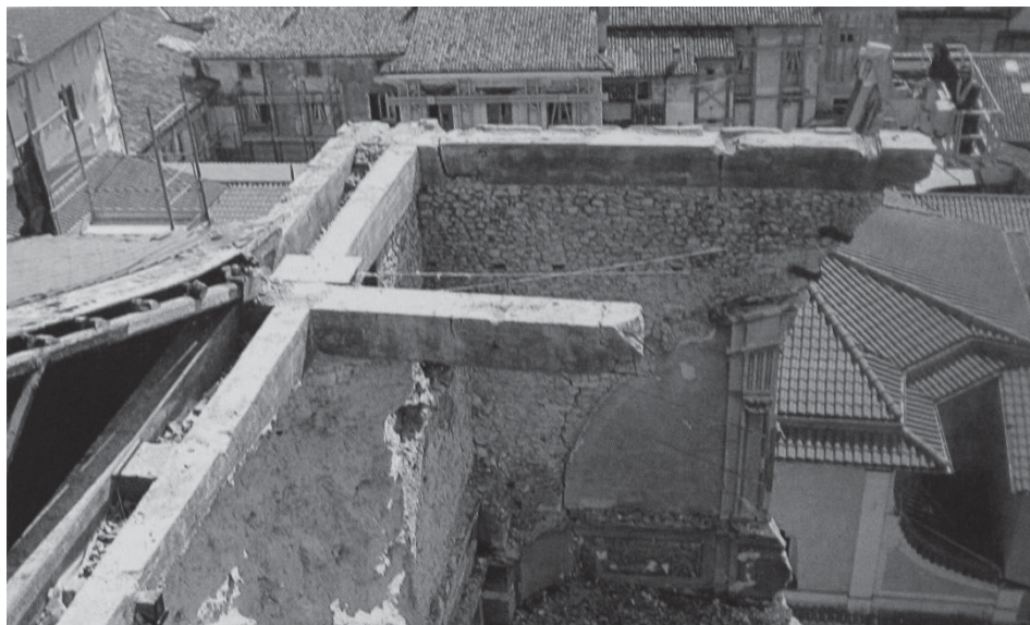
Fig. 5.3 Cathedral of San Massimo after the quake event of 2009. After the collapse of the dome, there is still present the top beam in reinforced concrete.
