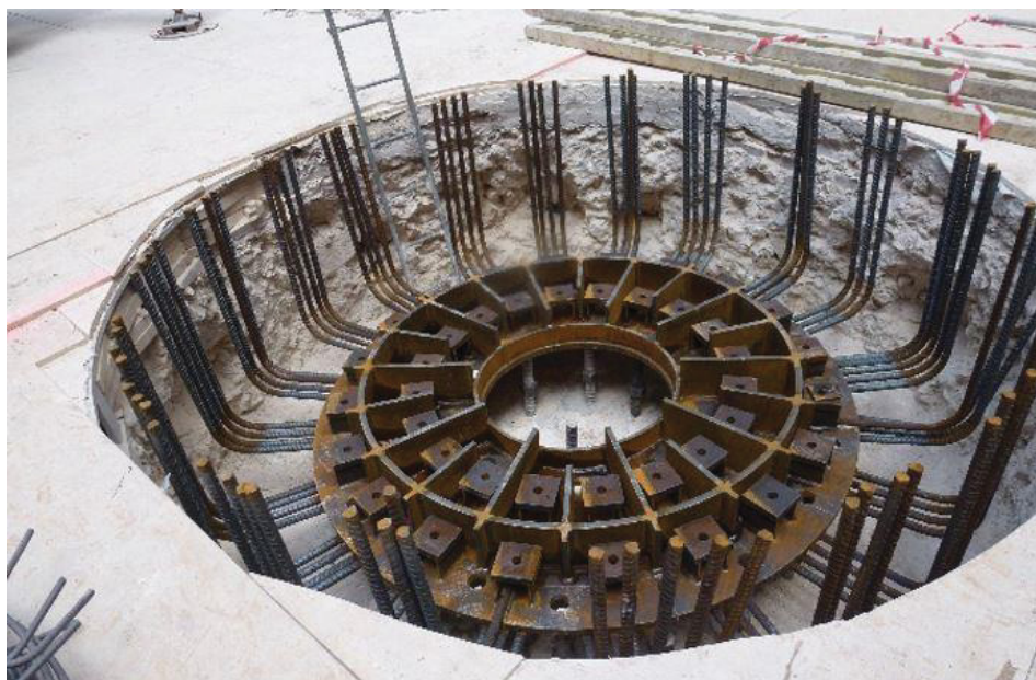
Fig. 6.1 The foundation of the new pillar in reinforced concrete of the reconstructed area.
