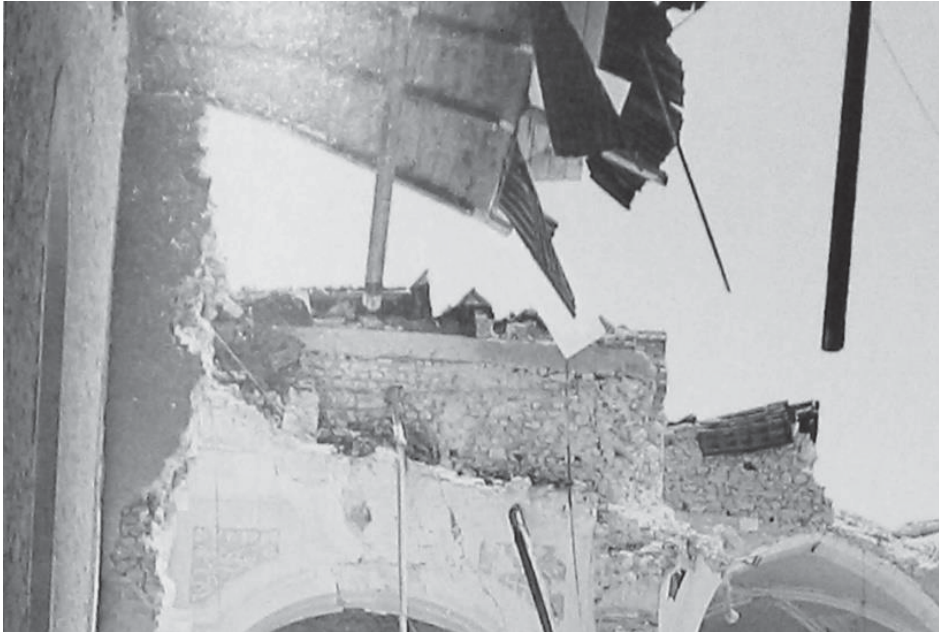
Fig. 5.18 The collapsed area of Collemaggio with the reinforced concrete elements hanging and the top beams visible due to the detachment of the plaster.
