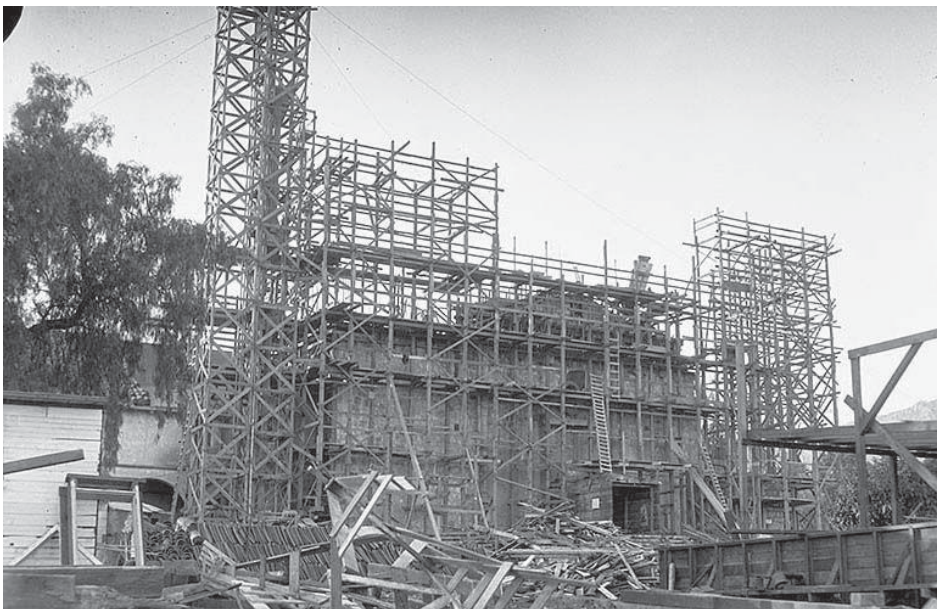
Fig. 4.32 Picture of Mission Santa Barbara during the restoration works, with the scaffolding in 1926 (UCLA).
