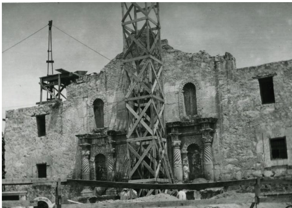
Fig. 4.20 The Alamo works of 1920 with the scaffoldings on the facade (photo from DRT)
