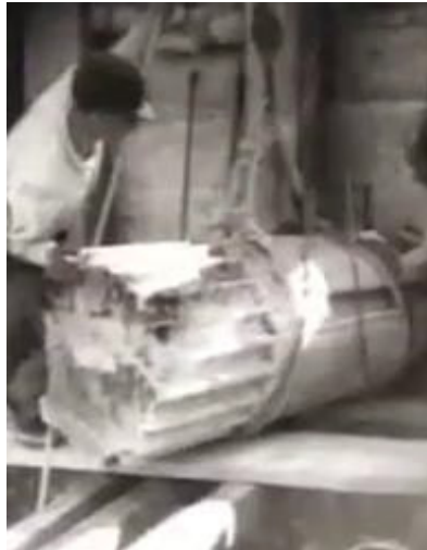
Fig. 3.74 - left The columns before be punctured for the insertion of reinforcement bars.
