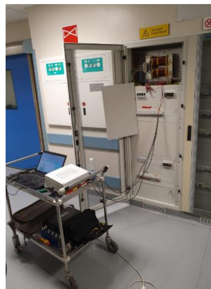
Fig. 3. SFRA test on isolation medical transformers of the hospital group 2 medical location
