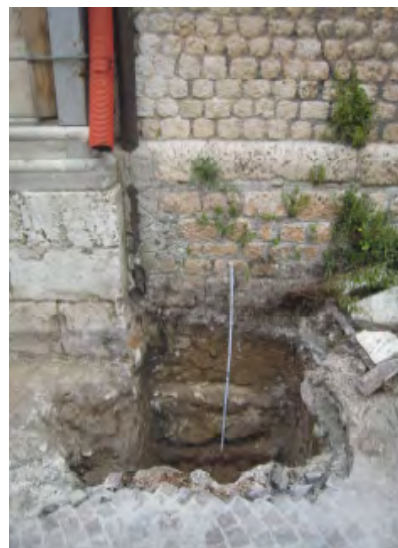
Figure 17. Photo of the inspection Pit, IP, near the foundation of the belfry, taken by Fine Art Authority.
