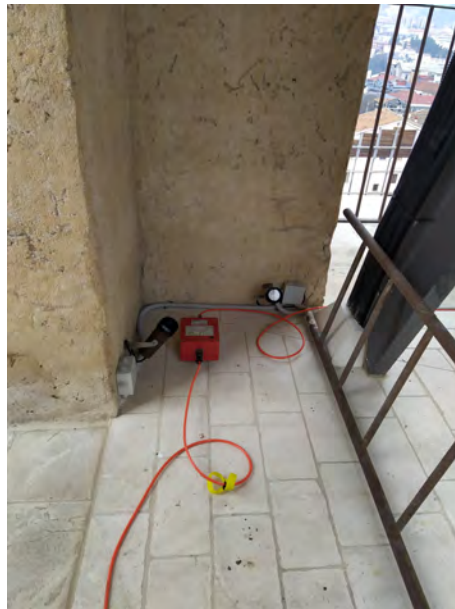
Figure 19. Accelerometer placed on the top of the bell tower, at the height of 22.03 m.
