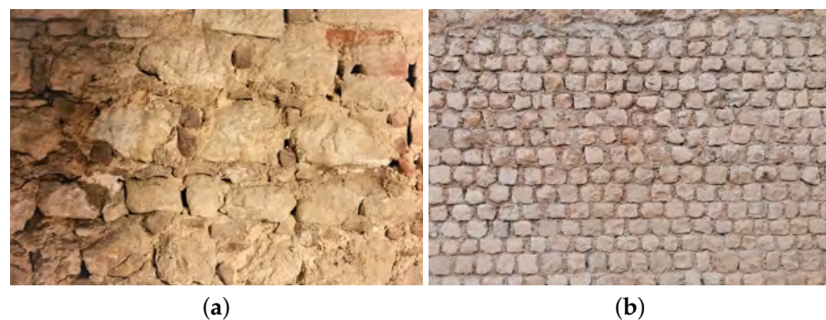
Figure 8. Texture of the masonry, after the restoration of the belfry (a) and of the nave wall (b).
